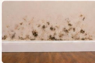
Mold behind walls
